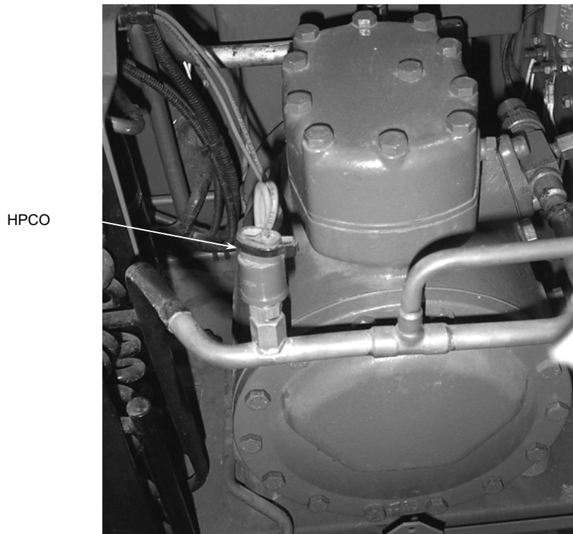
Figure 1. High Pressure Cutout Switch (HPCO).
