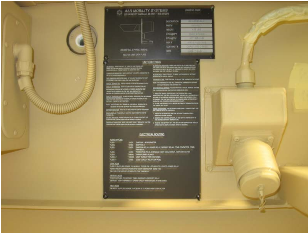
Figure 12. Photo of the Refrigeration Unit and Unit Controls Placards.
