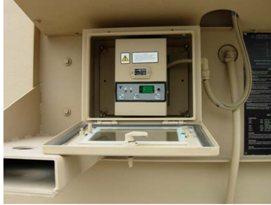
Figure 1. RU Electrical Enclosure.
